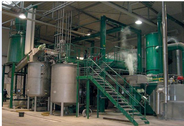
FLOTTWEG SORTICANTER® system for the recovery of polyolefins from mixed plastics at a German company
